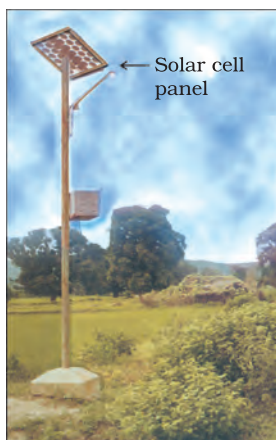
Figure 14.7 A solar cell panel
